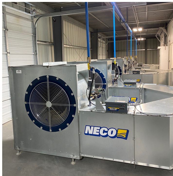
New burner blower fans (Mabton Ranch)
