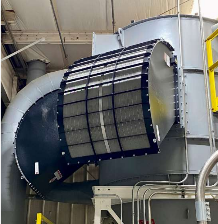
New dust abatement filter
